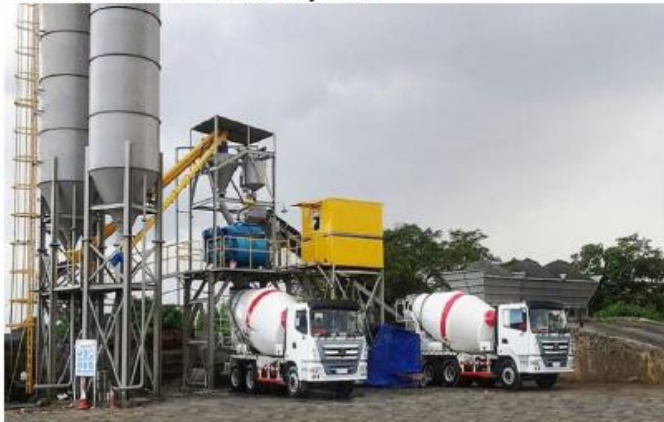
Gambar 2. Fasilitas Ready mix
